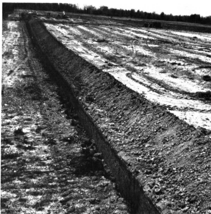
Figure 6. —Installation of a subsurface drainage system to remove excess water from Capac loam, 0 to 3 percent slopes.
